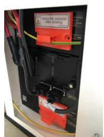
Battery terminal connections:
