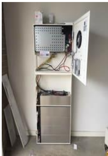
Battery module positioning:
